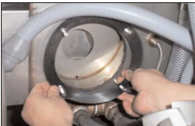
Removing the pump gasket
