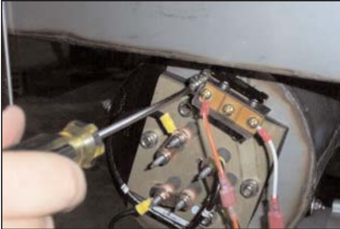
Calibrating the new thermostat.
