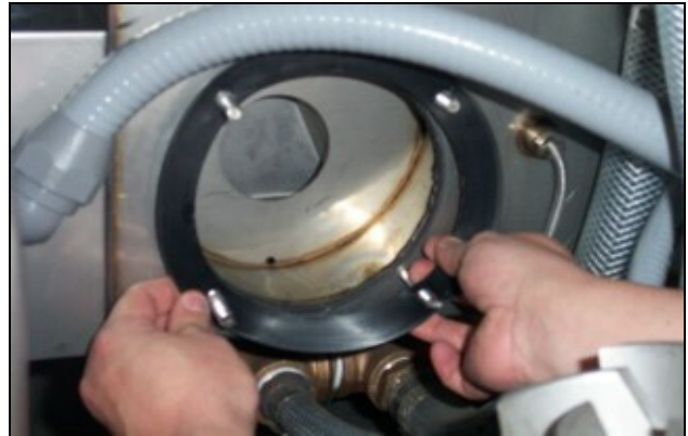
Removing the pump gasket
