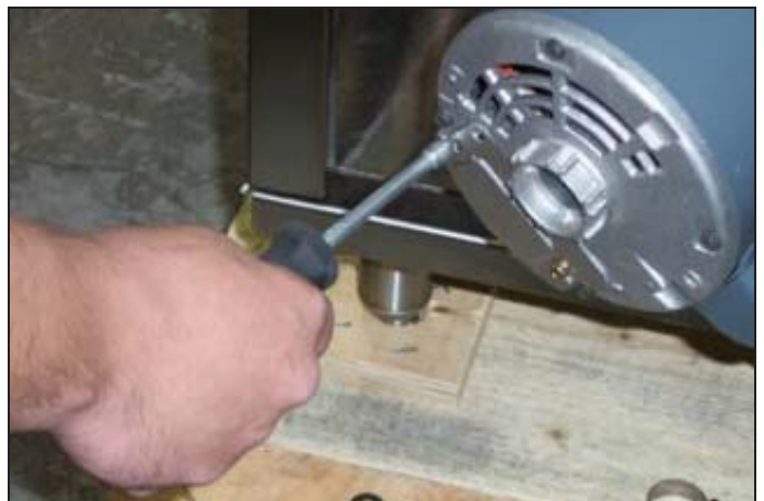
Removing the wiring cover.
