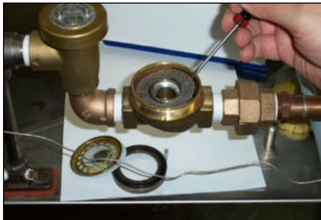
Removing the mesh strainer screen
